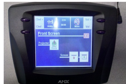
Figure 1 The AMX control panel
